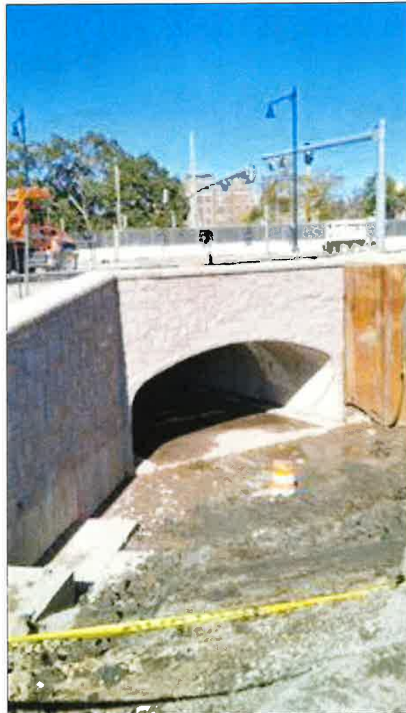
Figure 37. Example of a culvert similar in size to the proposed Peckman River diversion culvert.
