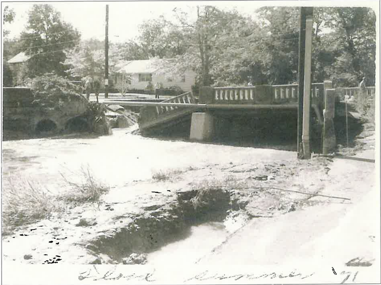
Figure 20. Damage from Hurricane Doria to a bridge abutment & road along the Peckman River (1971).
