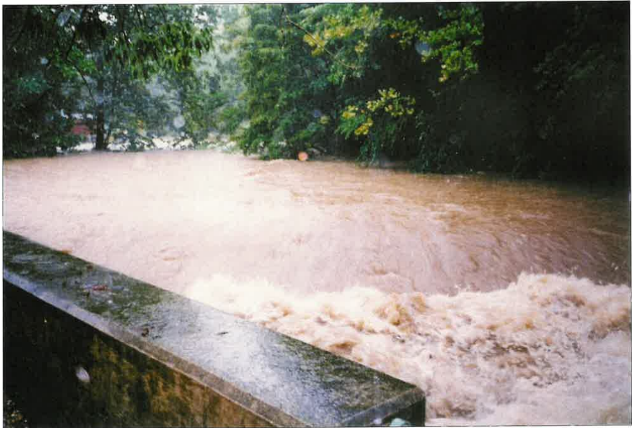
Figure 21. High flows and water levels due to Hurricane Floyd at a bridge abutment along the Peckman River (1999).
