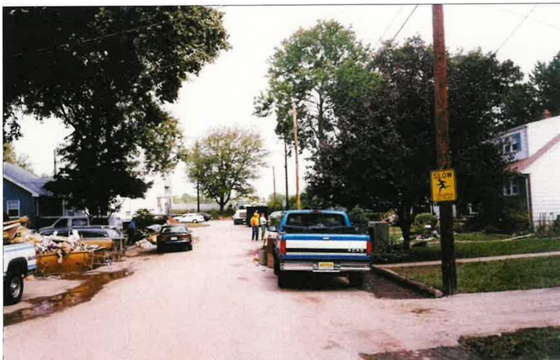
Figure 12. Repairs being performed on a property due to Peckman River flood damage from Hurricane Floyd (1999).
