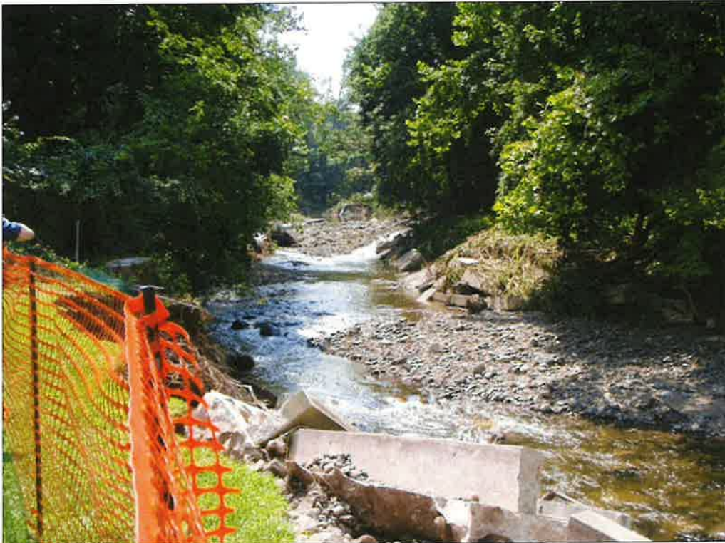
Figure 23. Peckman River erosion in Little Falls, New Jersey (August 2018).
