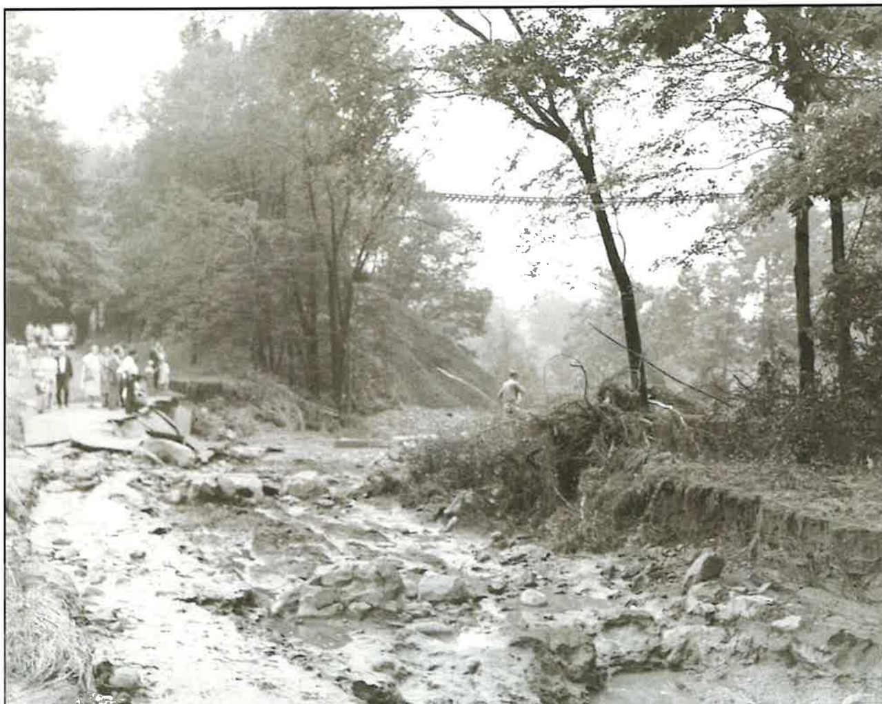
Figure 18. Erie Railroad tracks suspended in the air after the Peckman River flood of July 1945 washed away the earth supporting the bridge for the tracks. Courtesy of the Little Falls Historical Society. Photographed July 22, 1945.
